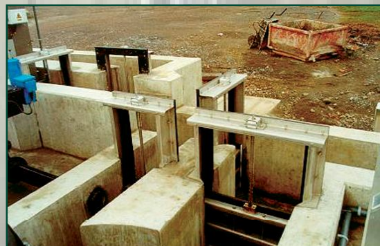
PKS sluice gates in Balaghaderreen wwtp Ireland
