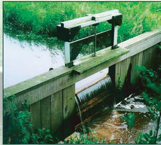
DPOS overflow gate in Soest Holland
