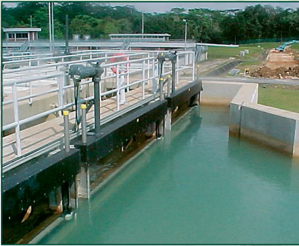
POS overflow gates in Chestnut wwtp Singapore
